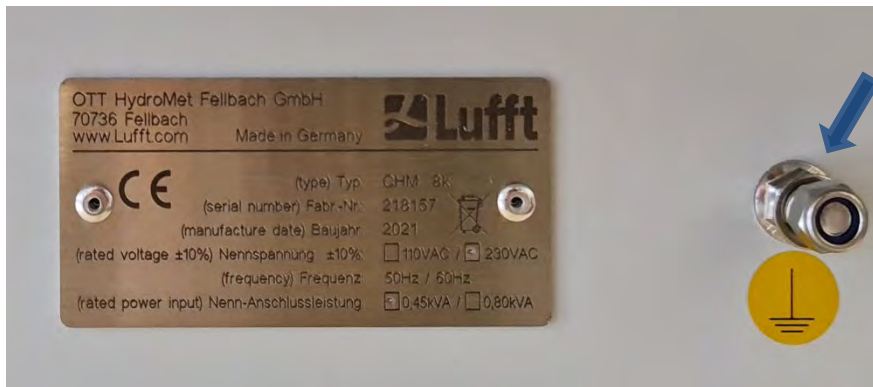
Figure 12 Grounding connection at pedestal of device.
